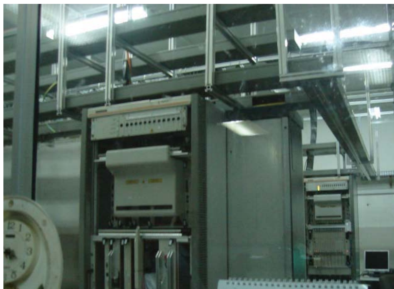
The SAT-3 fiber optic cable makes landfall in Nigeria in the Nitel headquarters in Lagos (above). The building also houses the NIXP domestic internet exchange. The building lacks a reliable power supply, modern security system, and proper climate controls for the equipment.
